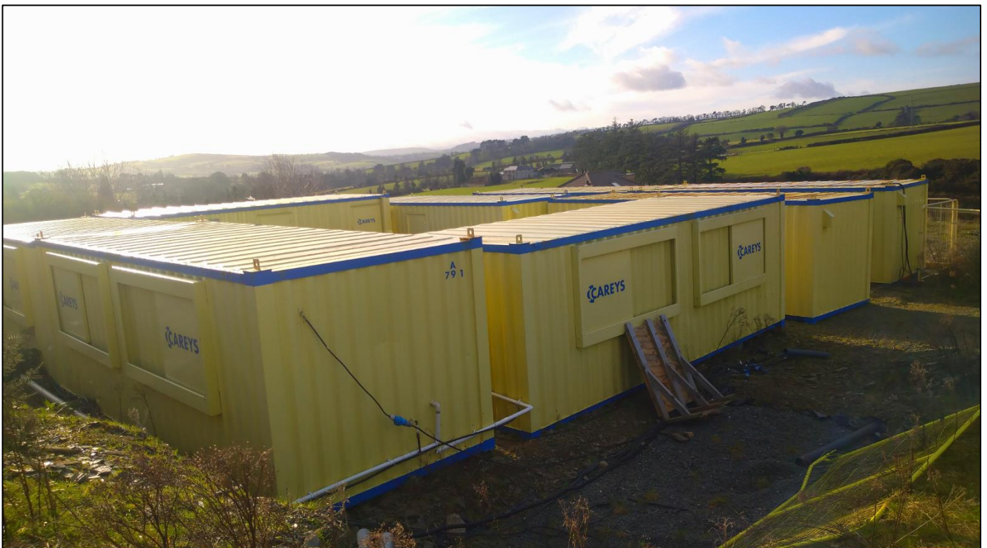
Plate 2: Steel cabins at the southwest corner of the site, note the depth of ground reduction to accommodate the cabins.
